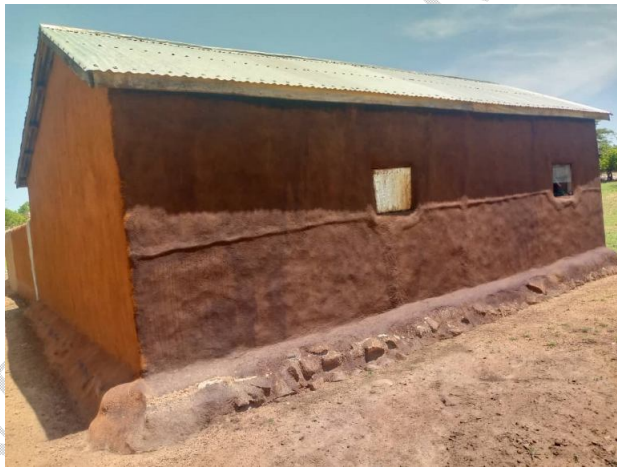
Figure 5: Back view of Plastered mud walls of rooms using mud mixed with Parkia biglobosa husk extract (Source: Personal fotos)
